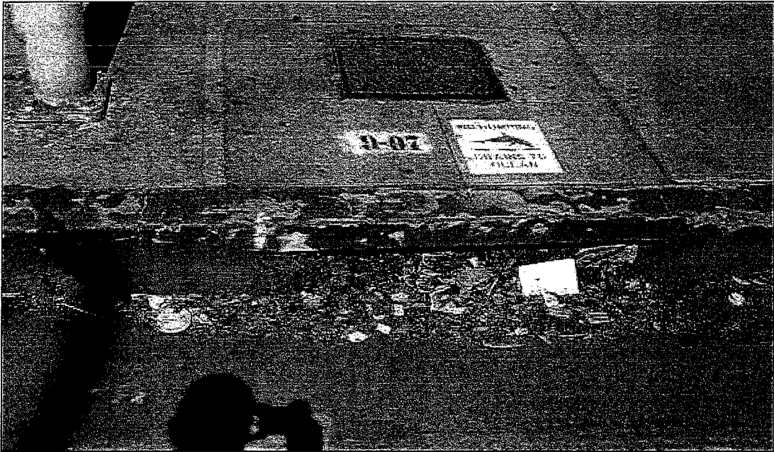
This excluder is stuck closed with trash and debris occluding the screen. According to local residents the area experiences local flooding issues in wet weather.
