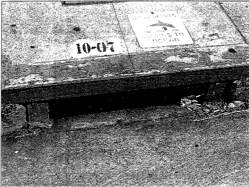
Excluder stuck partially open apparently not due to trash wedged in the opening.
